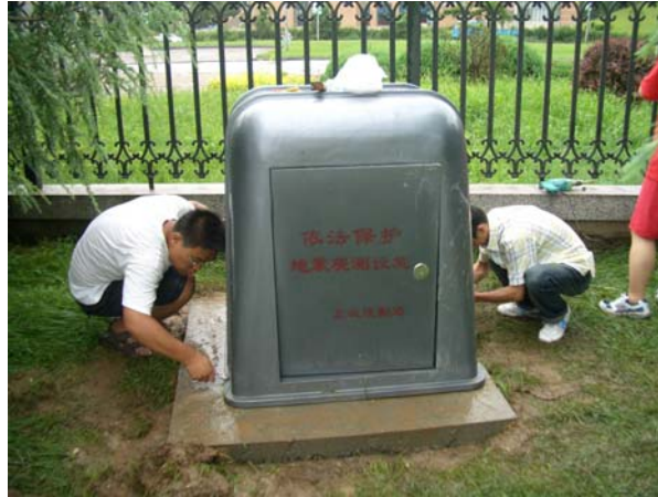
Fig.7 Installation of the instrument housing on free field site in the front of ICC
